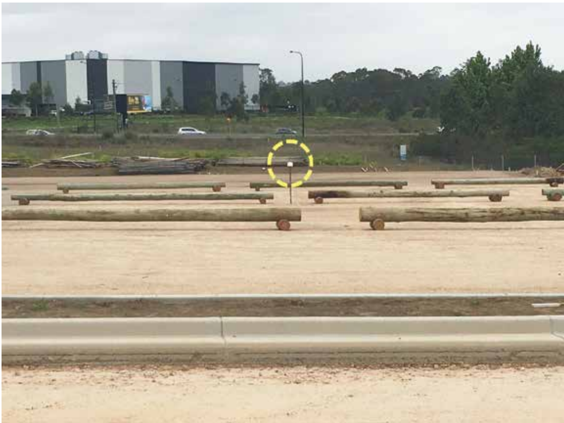
FIGURE 8: Example of positioning TinyTag logger in the open space of the overflow car park (location B) in October 2018. At that time, uncovered subgrade made up the surface of this site and also that of the main car park. Image © S. Pfautsch
