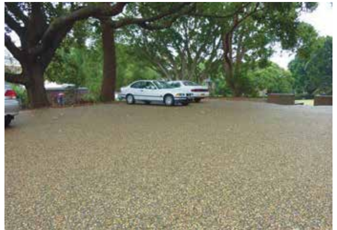
FIGURE 38: Example of resin mix (SuperStone™ from MPS Paving Systems Australia, www.mpspaving.com.au ) applied to a car park at the University of Sydney. Image © SPEC-NET ( www.spec-net.com.au ).
